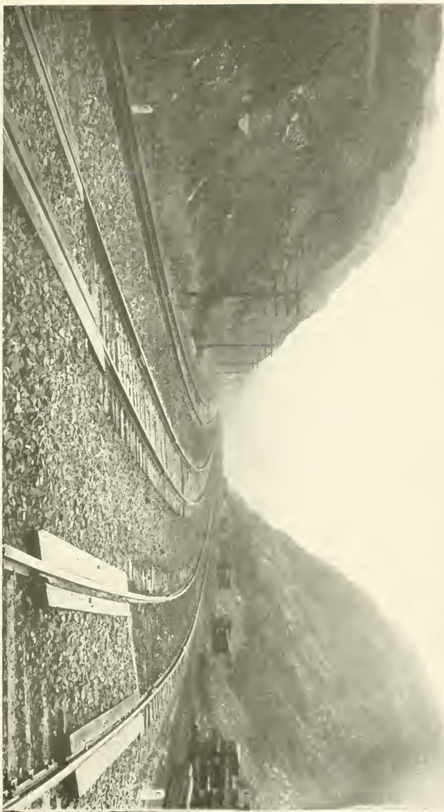
View of the three-track line of the Baltimore and Ohio Railroad in Preston County, showing the open cut which has taken the place of McQuire's tunnel.
